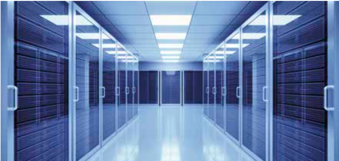
Data centre cooling
